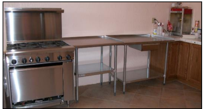
New 6 burner gas stove & tables will enable the people to provide food for the community.
