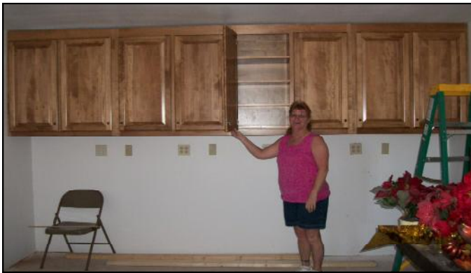
New cabinets installed in classroom. Made by Sclabach Wood Design of Baltic, Ohio.
